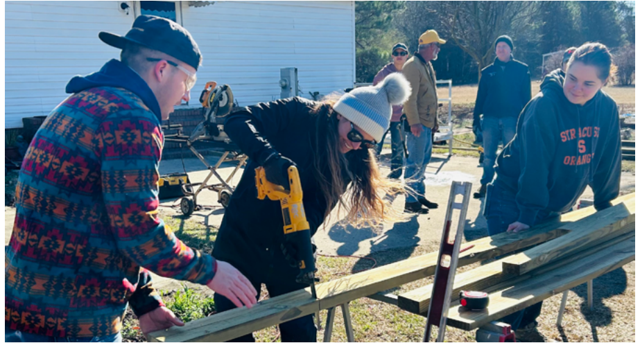
Volunteers from five Twin Cities churches work together to build handicap ramps while on mission in North Carolina.
